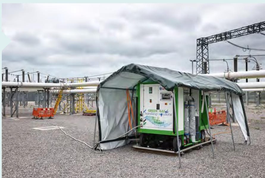
Onsite gas cart used to retro fill existing gas-insulated, high-voltage switchgear, with an alternative low global warming g 3 gas, designed for high-voltage transmission equipment, Richborough Substation, Kent, UK
