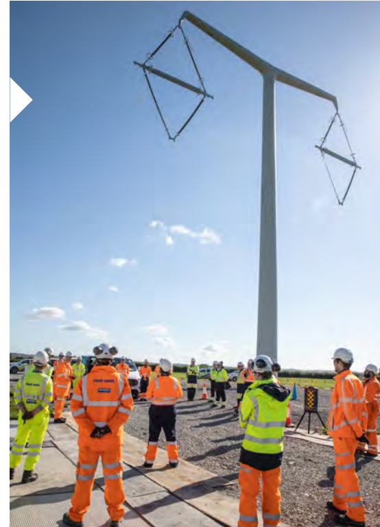
The first of 53 T- pylons, erected in September 2021 as part of the Hinkley Connection project in the UK
